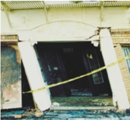
Figure 4.45 How could an engineer design buildings so they would not bend or buckle during an earthquake?
