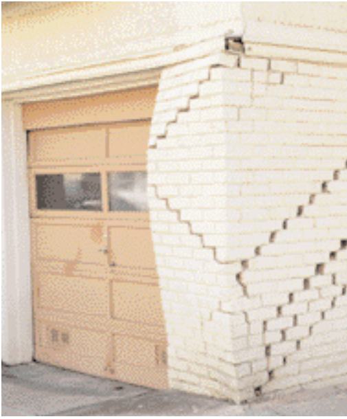
Figure 4.44 Even if the ground beneath a building was uniform when the building was constructed, shear damage can occur. An earthquake caused this damage.
